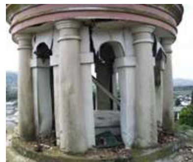
Figure 7-10 1999 Earthquake Courthouse Damage
